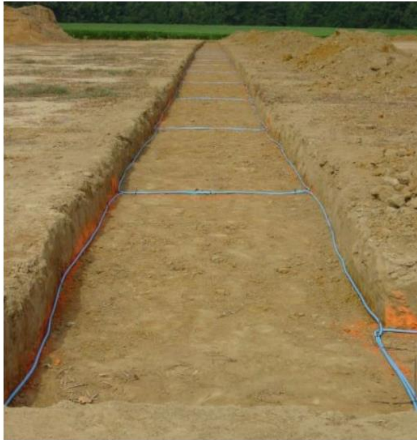
Figure 49. Cabling Hardware for UGS
